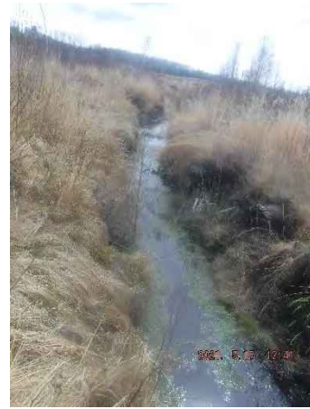
Photo 6: Ditch looking north, slumping along ditch.
