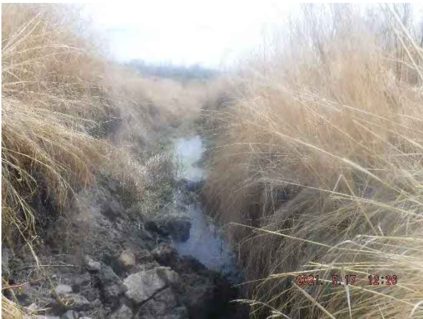
Photo 7: Erosion/slumping within ditch
