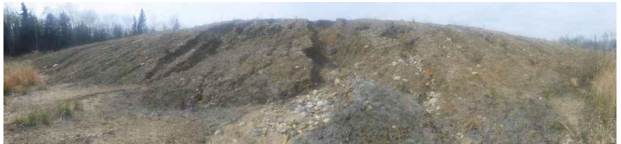
Photo 3: Erosion along the south boundary
